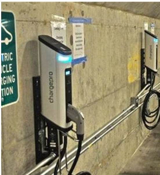
Electric Vehicular charging stations in an underground parking lot
